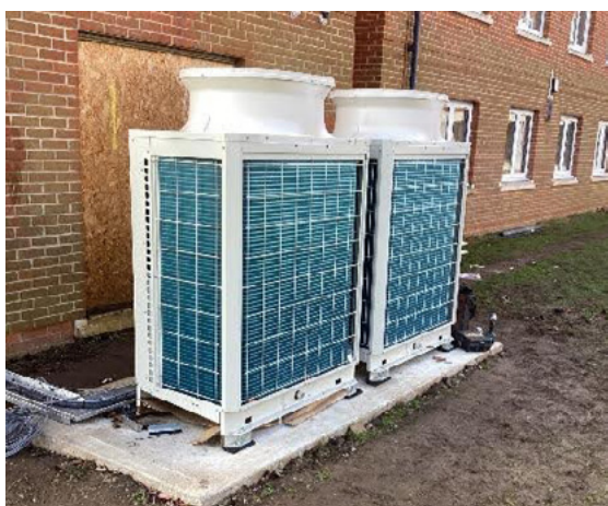
Air source heat technology at Langstone Campus.
